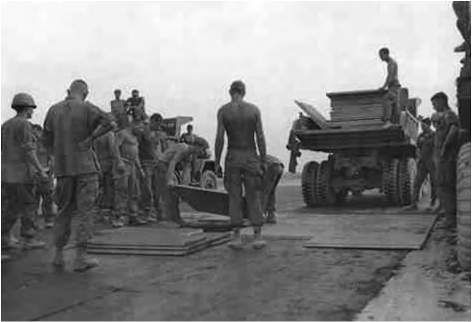
Men of the 39th Engineer Battalion lay MX19 matting at Duc Pho.
